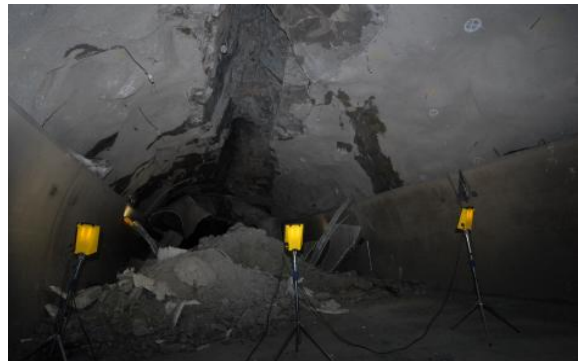
Figure 1. Rockfall in Hanekleiv tunnel
