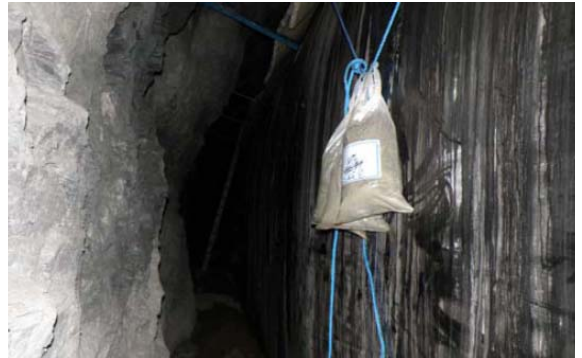
Figure 6. Bags with wet sand placed on the inside of the protective wall
