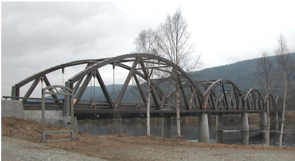
Figure 1: Evenstad Bridge in Norway (1996) is designed for full traffic load and has a length of 180 m
