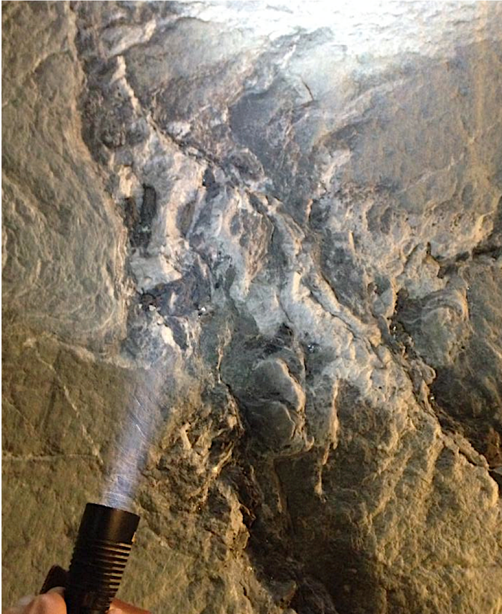
Figure 11. Observation of pegmatite with large elements of mica, Picture taken in the TBM-tunnel during site visit.
