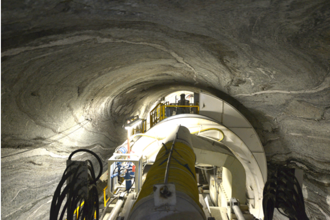
Figure 9. The geology in the TBM-tunnel. The picture is taken in the TBM-backup and backwards, during site visit.
