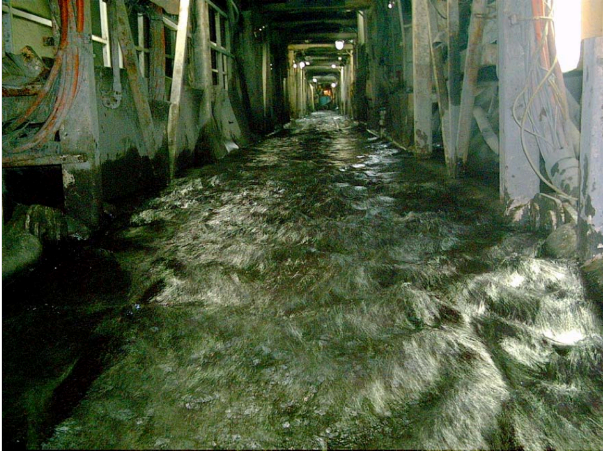
Figure 30. Water inflow with estimated leakage of 800 l/s in the TBM backup (Wenner & Wannemacher, 2009).
