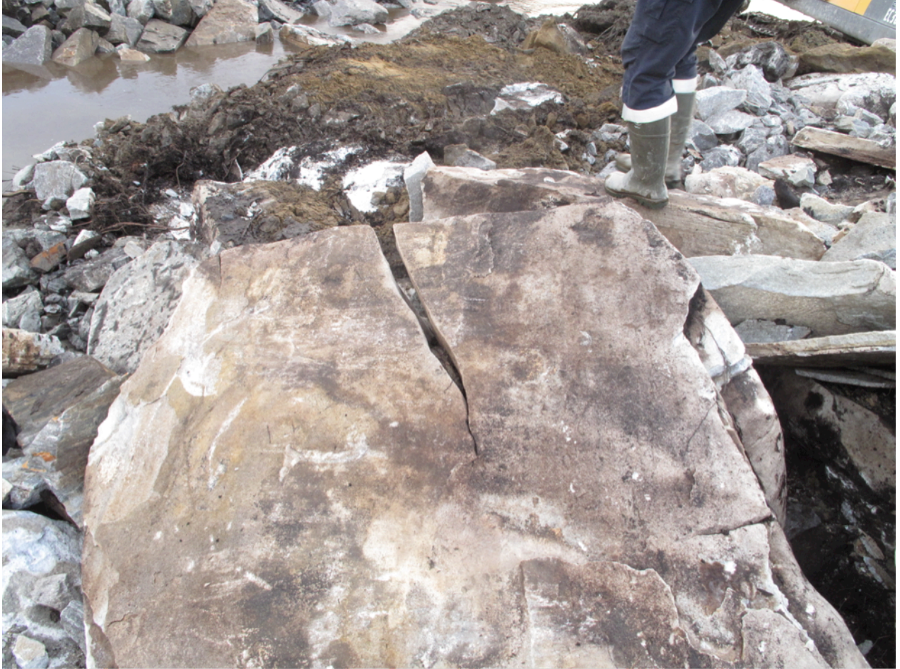
Figure 16. Solution of joint in marble at the construction area for the planned intake at Fallfors. The photo is taken by Erik Dahl Johansen in October 2013.
