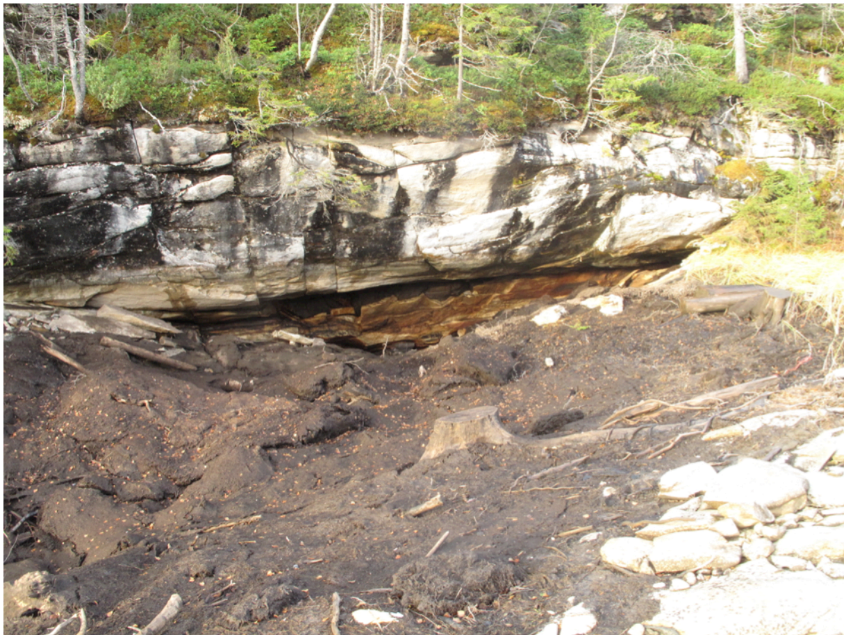
Figure 15. Solution of joints in marble at the originally planned intake at Fallfors. The photo is taken by Erik Dahl Johansen in October 2013
