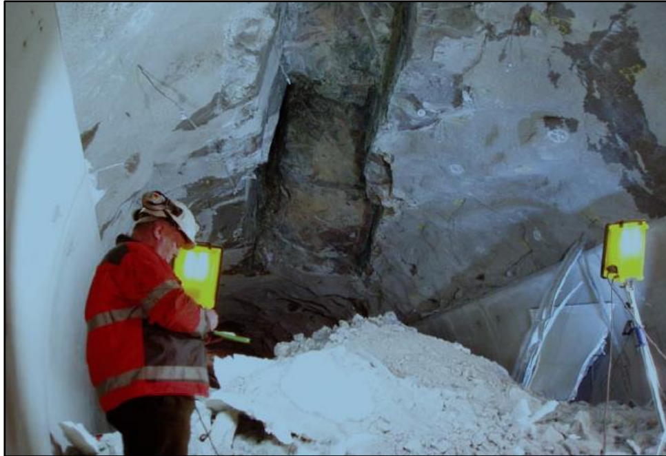
Figure 3-13: Photo of the collapsed area in the roof of the tunnel and the material from the cave-in on the floor of the tunnel (Nilsen, 2012).
