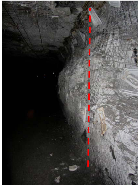
Figure 6.6 The pillar between main tunnels of the mine located in front of the panel C6. The location of the pillar is shown in Figure 6.5.
