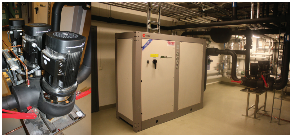
Figure 1.3 Circulation pumps for borehole heat exchangers (left) and ground-coupled heat pump at Nardo school (Trondheim, Norway).
