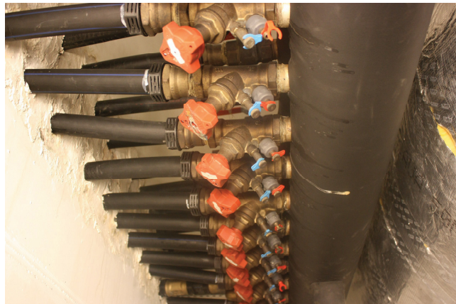
Figure 1.4 Borehole heat exchangers entering the HVAC (Heating, Ventilation, Air-Condition) centre at Nardo school (Trondheim), 14 boreholes.
