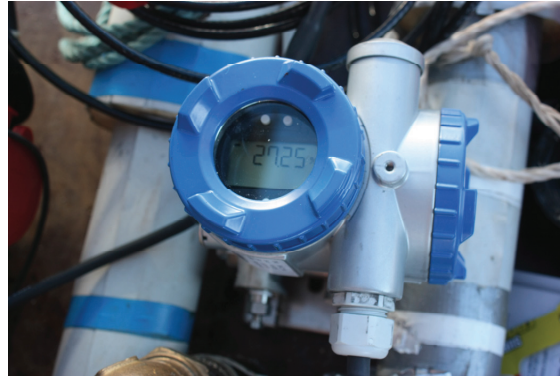
Figure 2.11 Differential pressure transmitter installed on the TRT trailer.
