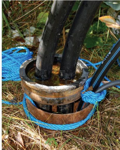
Figure 2.4 Borehole at Lade equipped with borehole heat exchanger (single U) and tube and electricity cable for the groundwater pump installed at the bottom of the borehole.
