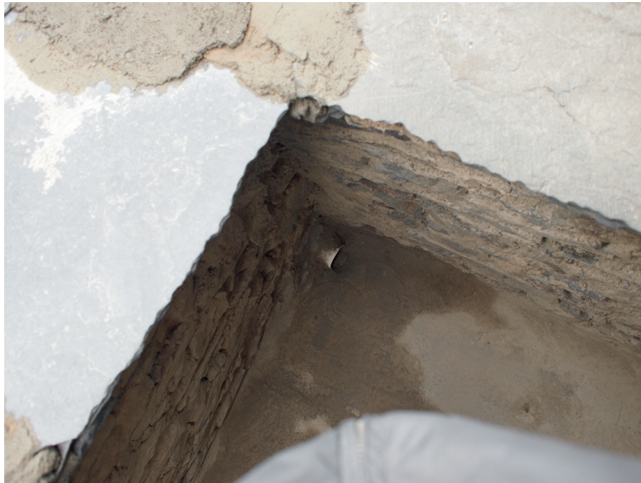
Figure 6. 8 Water Leakage on the Roof
