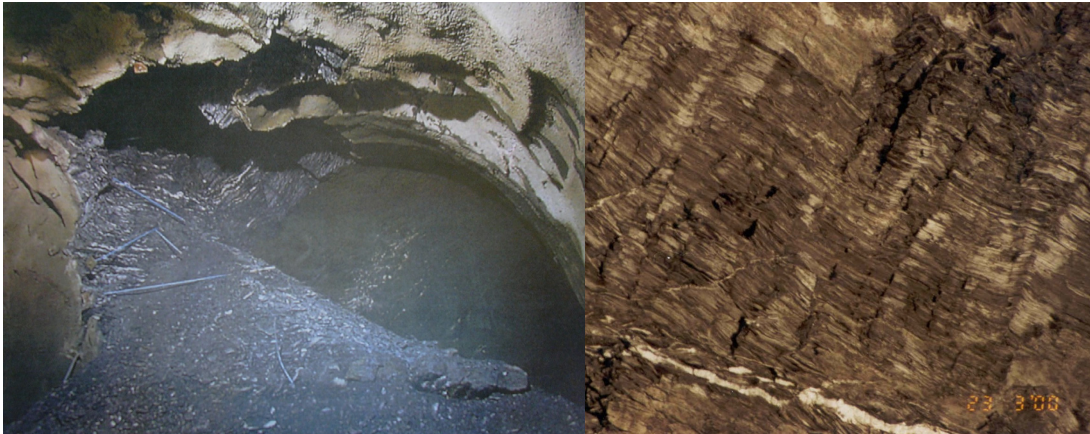
Figure 1-5. Headrace tunnel collapse at Kaligandaki “A” Hydroelectric Project (left) and tunnel face showing thin foliation plane with very weak bond (right) (Photo: Impregilo SpA, 2000).
