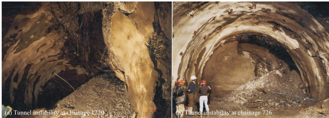
Figure 4-10. Collapse due to strength and stress anisotropy (left) and cracks formed by high squeezing pressure (right) (Photo: Impregilo SpA, 1999).
