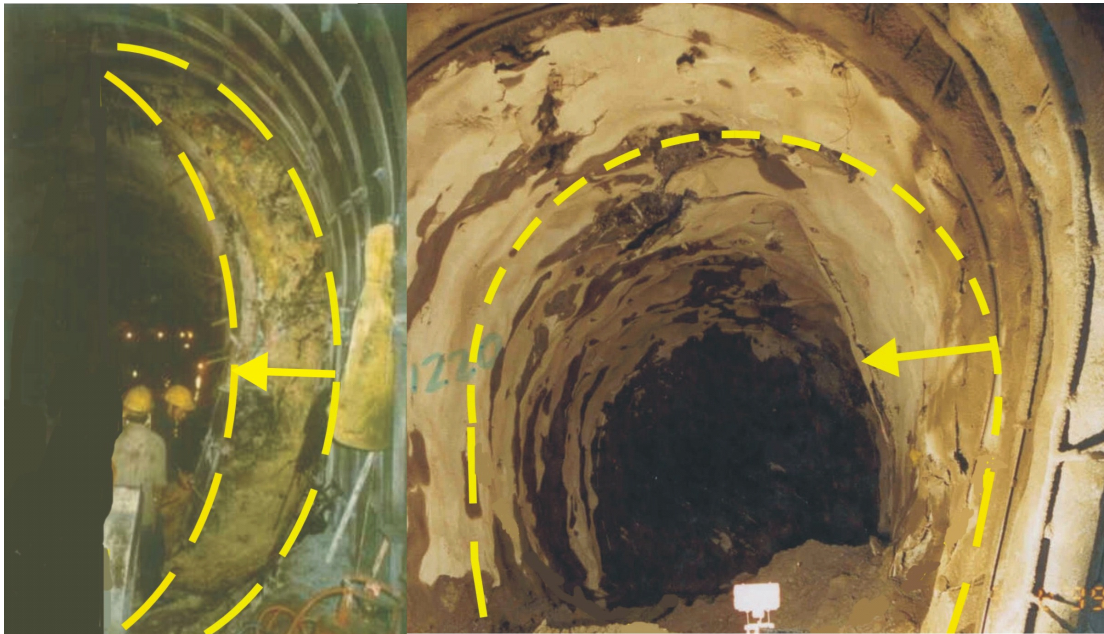
Figure 1-8. Severe squeezing at Modi pressure tunnel (left) and Kaligandaki headrace tunnel (right) (Photo: Himal Hydro, 2001 and Impregilo SpA, 1989)
