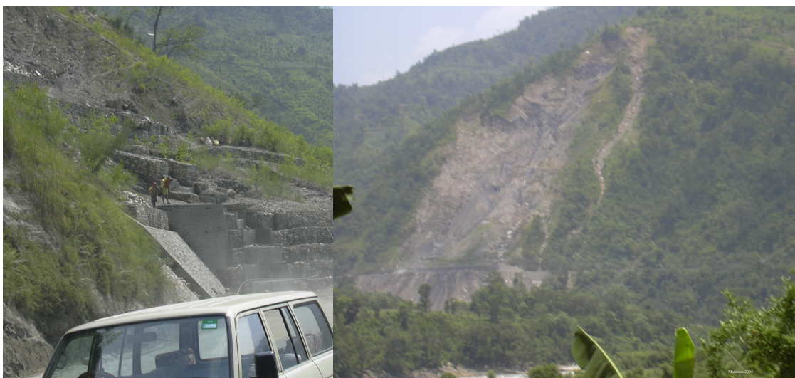
Figure 1-4. A major slide at Krishnavir along the Prithibhi highway “a main gateway to Kathmandu valley”. Slope protection works with gabion (left) and the extent of slope failure (right).
