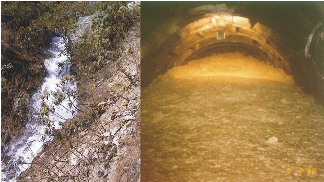
Figure 1-9. Water leakage from Adit 2 of Khimti headrace tunnel after early water filling (left) and mass inflow of water mixed with debris from a shear fault at the pressure tunnel of Modi Khola (right) (Right Photo: Himal Hydro, 1998).
