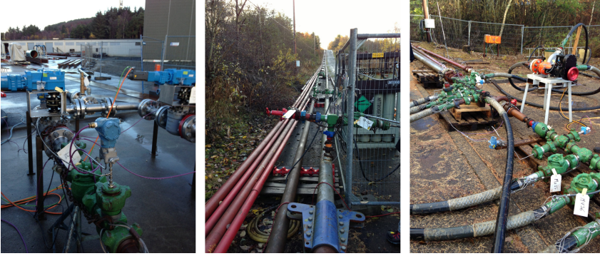
Figure 4.2: Experimental flow loop with choke manifold to the left, gas influx and washout emulsion in the middle, and bit and loss emulation to the right.
