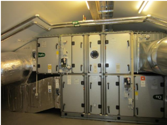
Figure 45 - Air handling unit
