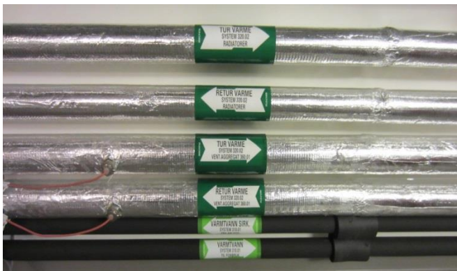
Figure 42 – Pipelines for heat distribution
