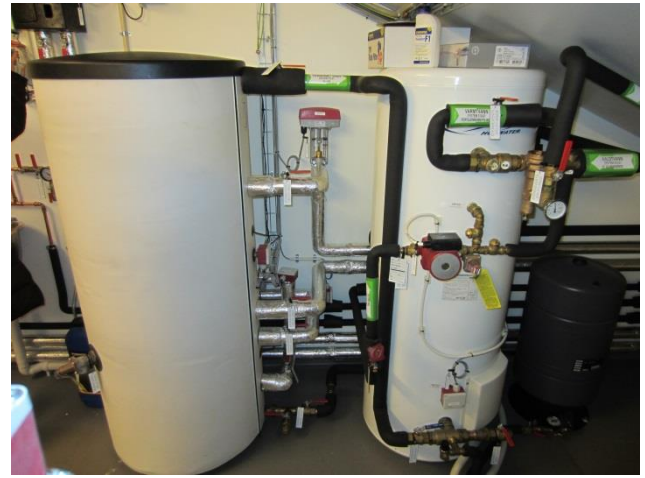
Figure 38 – Tap water heaters: preheating and additional heating
