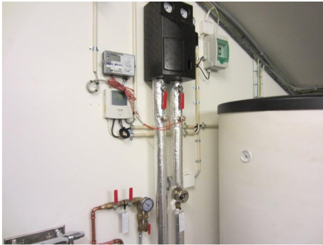
Figure 37 – Solar collector pump and measuring instrument
