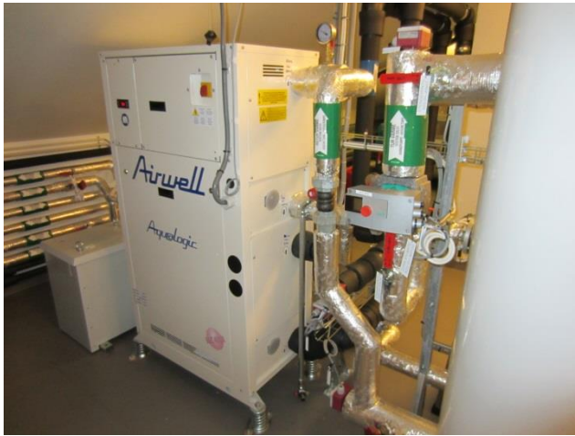
Figure 33 – Heat pump of brand Airwell
