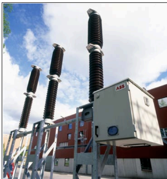
Figure 6 Live tank Circuit Breaker type LTB 145D (ABB, 2004)
