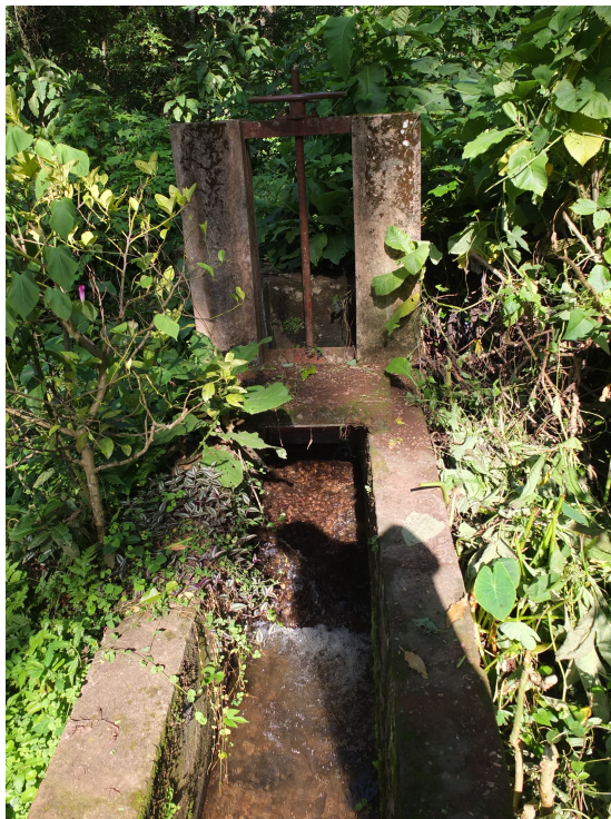
Figure 4.7: Channel and gate valve at turbine level.
