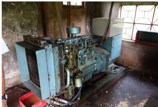
Figure 4.12: One of the three diesel generators.
