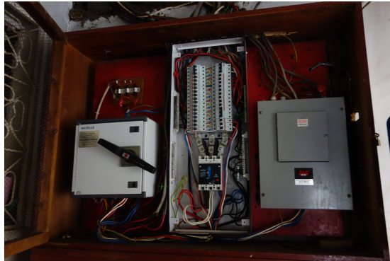
Figure 4.13: Main changeover switch.
