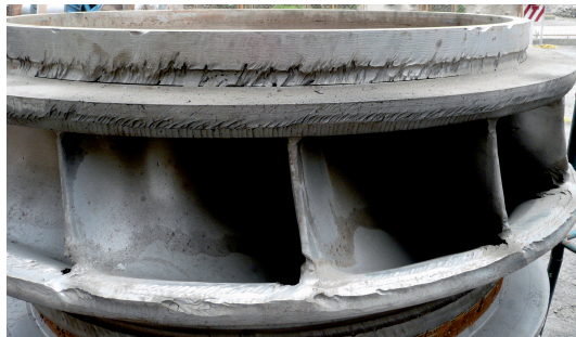
Figure 2.3: Eroded runner from Cahua Power Plant
