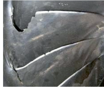
Fig.2 Erosion damage of Francis runner in Nepal
