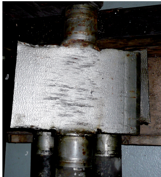
Figure 2.2: Guide vanes at Cahua Power Plant
