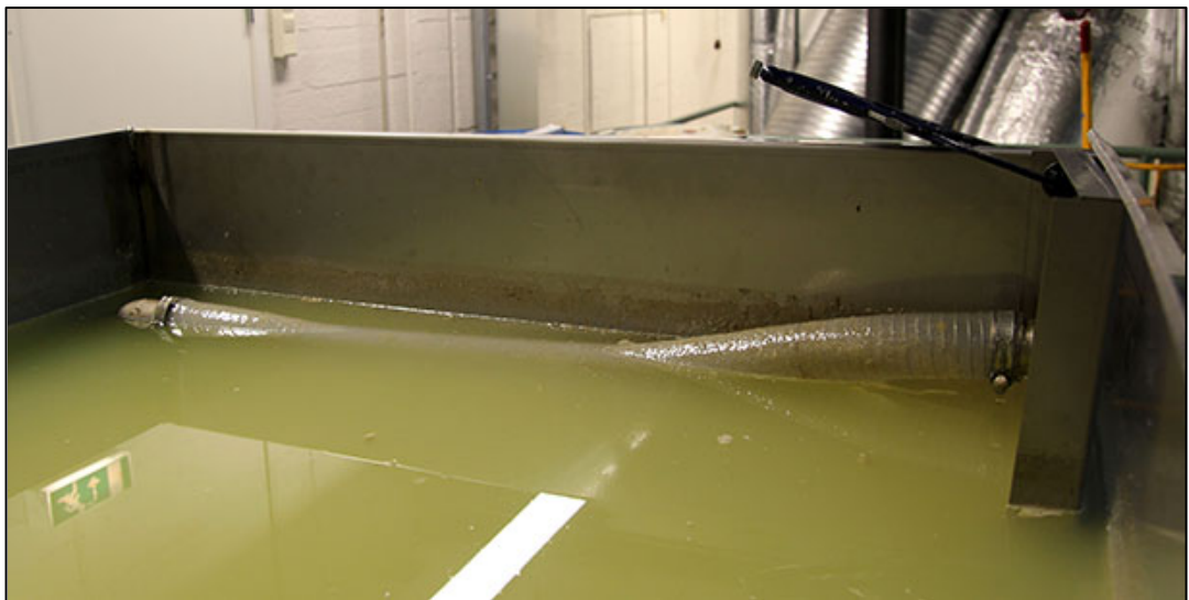
Figure 3.9 – Flexible flowline seen in low liquid level.
