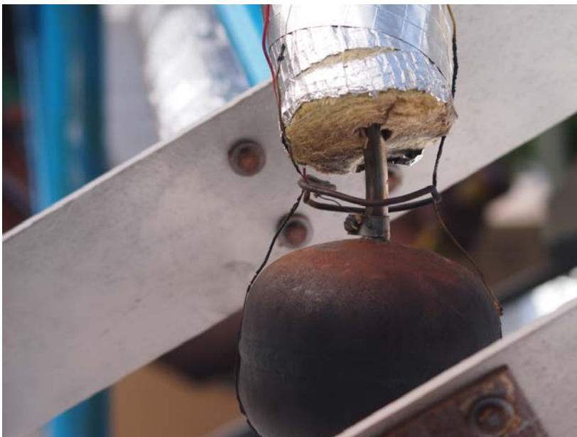
Figure 21- Boiler and steam pipe with insulation
