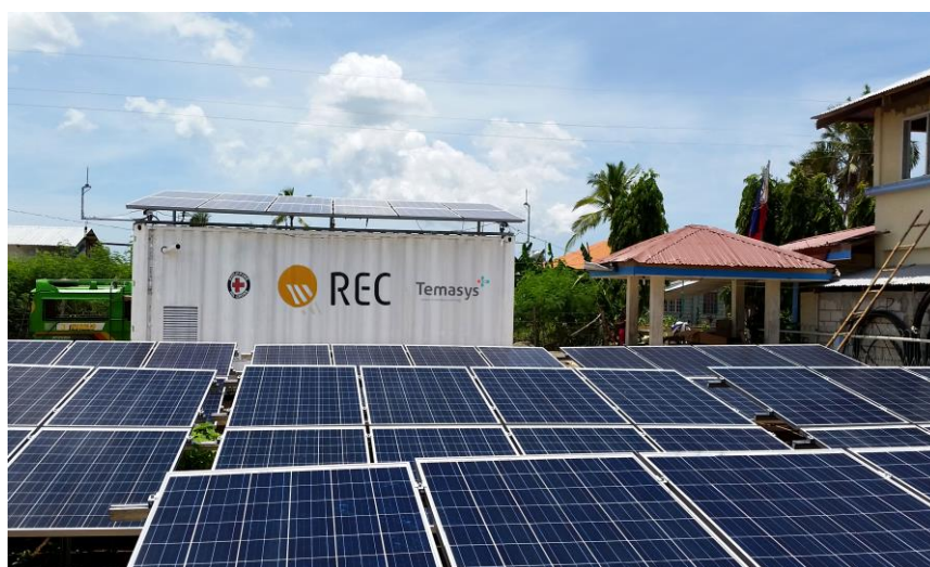
Picture 1. SolarBox Installation in Barangay Sungko, Bantayan. Photo: Vishal Vijay/REC.
