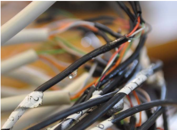
Figure 4.1 Leakage through wires
