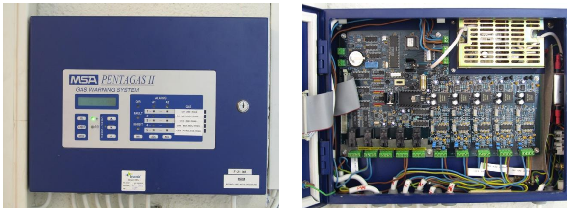
Figure A1: Overview of the Gas warning system (External and Internal views)
