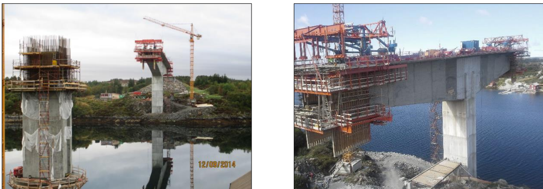
Figure 3.10 Dolmsundet bridge under construction. a) view from Dolmsundet towards Hitra [30] b) Cantilever with form traveller on the cantilever edges [31].
