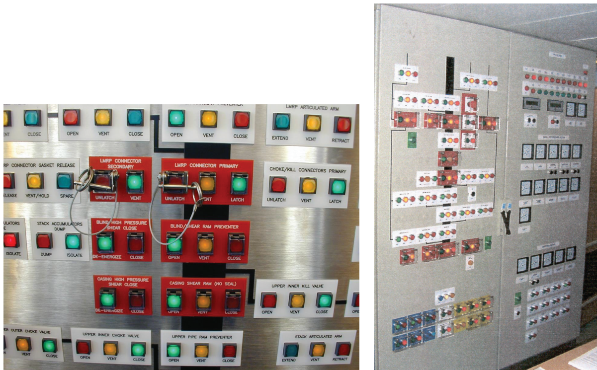
Figure 2.3: Driller's panel, from Imperial Oil and ExxonMobile (2009)
