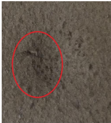
Figure 41: Cracks and spalling of sample 1
