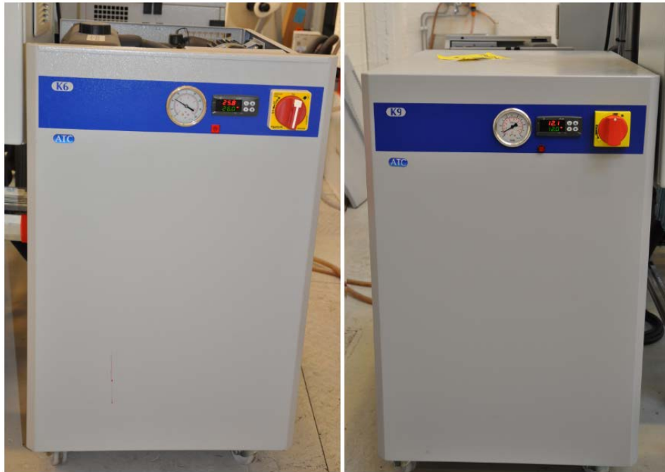
Figure 51: Heat exchangers (K6 on the left and K9 on the right)
