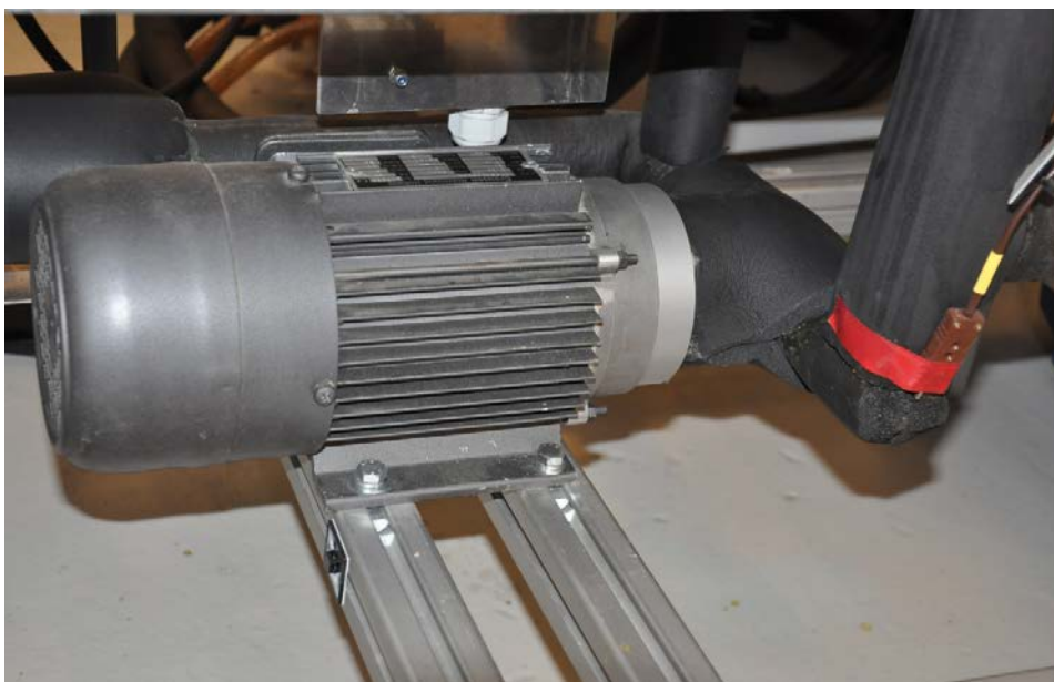
Figure 8: Pump with engine
