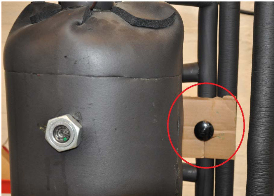
Figure 53: By-pass valve for pump
