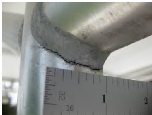
Figure 1.1: A tubular joint with crack developing
