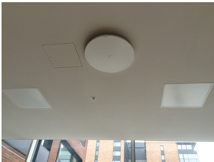
Figure 4.3: Air diffuser and radiators
