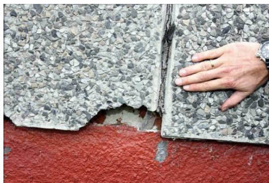
Figure 20. The façade in the West and East walls is worn out.
