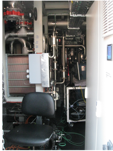
(b) View of the inside, with the VSD on the right and the green cables for the cylinder pressure transmitters out from the compressor on the floor
