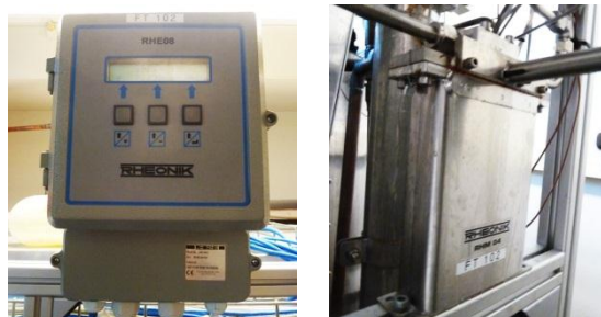
Figure 20: RHEONIK mass flow meter control panel, Mass flow meter installed in CO 2 loop.
