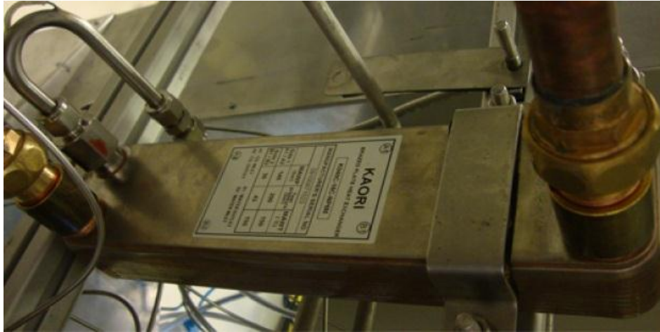
Figure 19: Picture of brazed plate heat exchanger.
