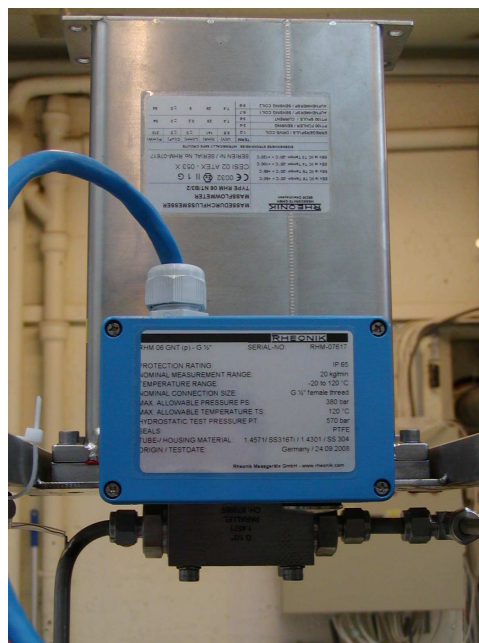
Figure 3.7: A RHEONIK RMH 06 mass flow meter installed in the heat pump loop
