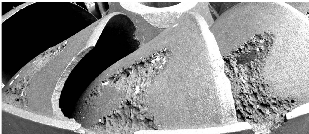
Figure 2.4: Severe cavitation erosion on a runner
