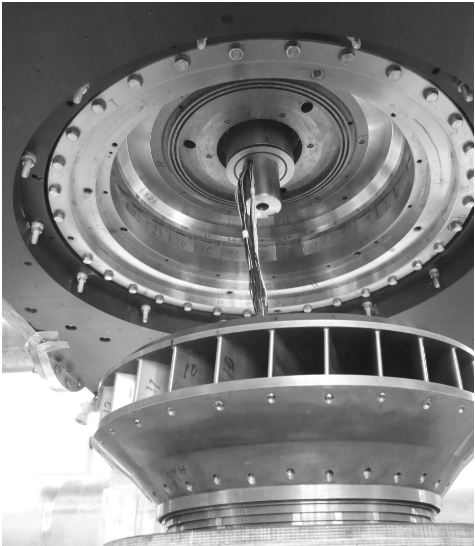
Figure 4 - Installing the instrumented NTNU runner. The cables from the sensors are run through the shaft.
