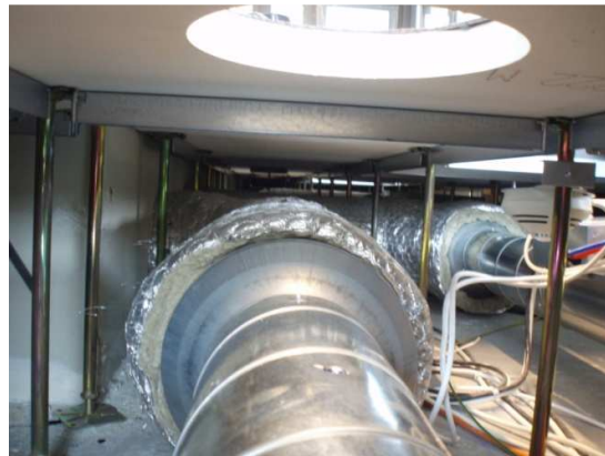
Figure 8.12: Fire insulation of supply ducts on the 5th floor.
