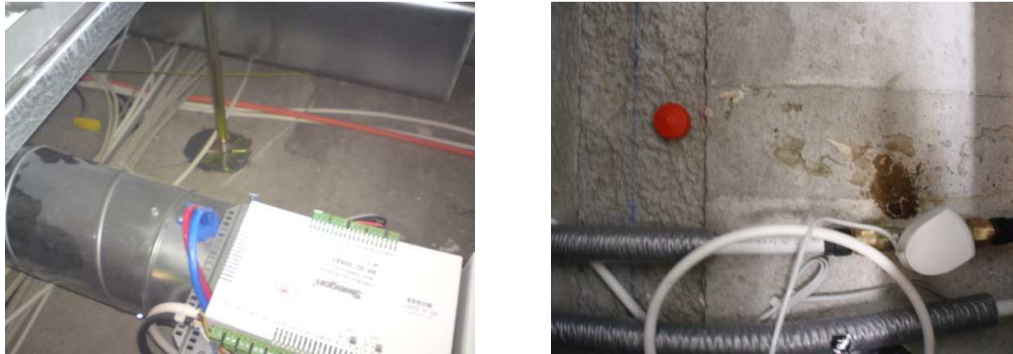
Figure 8.10: Dust and dirt in the underfloor plenum.
