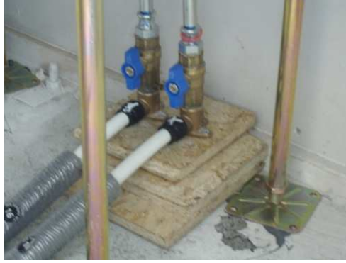
Figure 8.11: Pressed wood board panels supporting the radiator valves.
