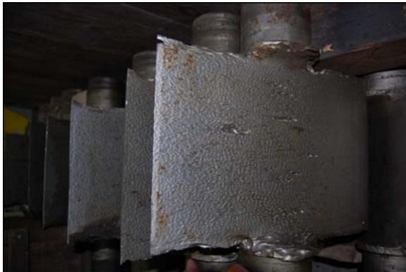
(a) Eroded guide vanes
