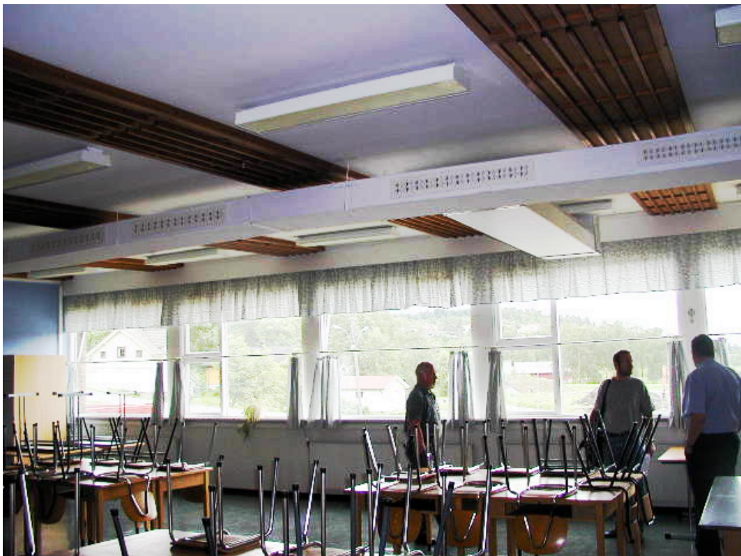
Figure 2. Thermally insulated air supply ductwork with integrated diffuser nozzles.
