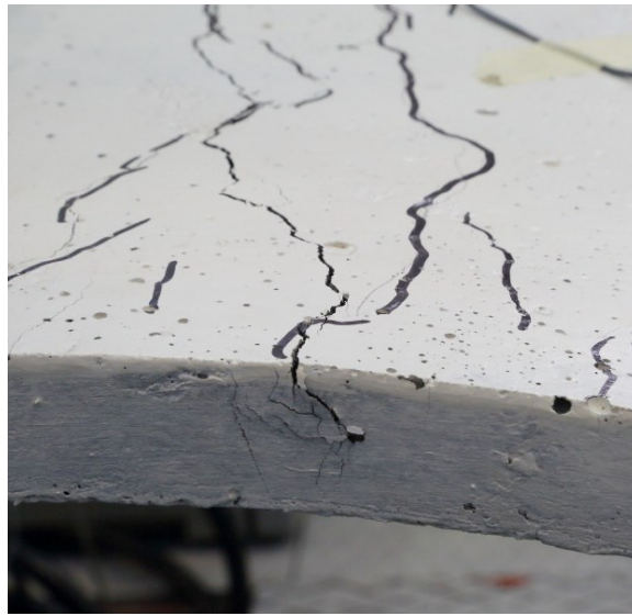
Figure 7.13: Cracking in area C (Figure 7.11)
