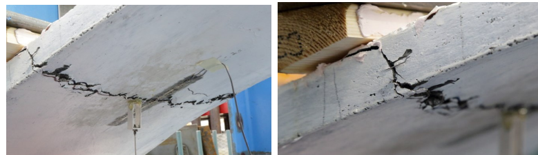
(a) Close view of crack under load (b) Prominent crack under load
