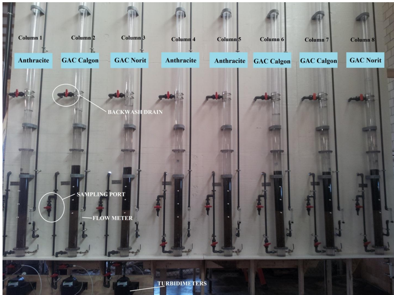
Figure 13: Picture of the filter columns of the pilot-scale filtration plant of MWW.
