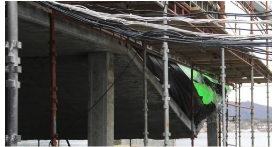
Figure 4: The test slab at the moment of collapse [12]
