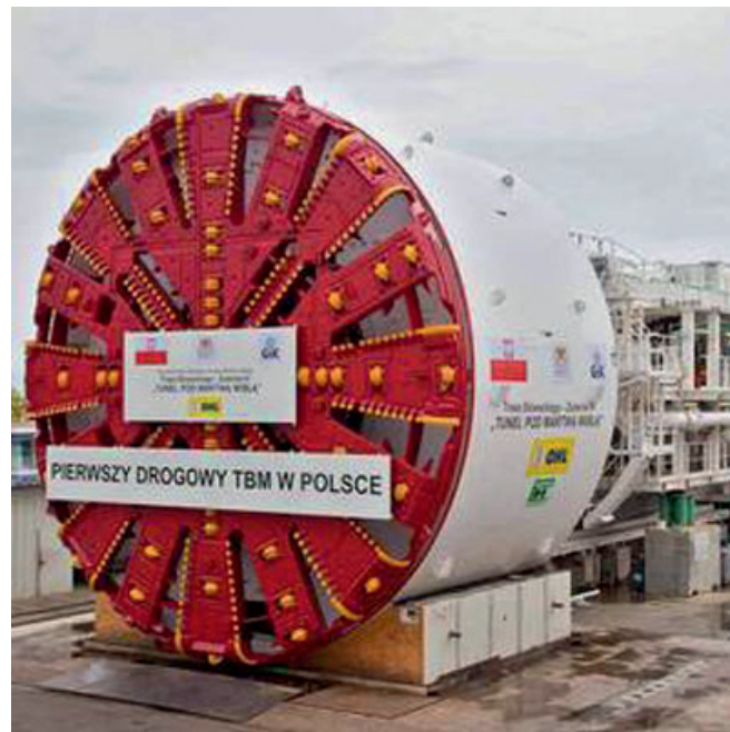
Figure 59. The slurry shield TBM being used to excavate the ongoing TBM project used for assessment of the validity of the estimators in the PhD study. (Photo taken from www.tunneltalk.com ).
