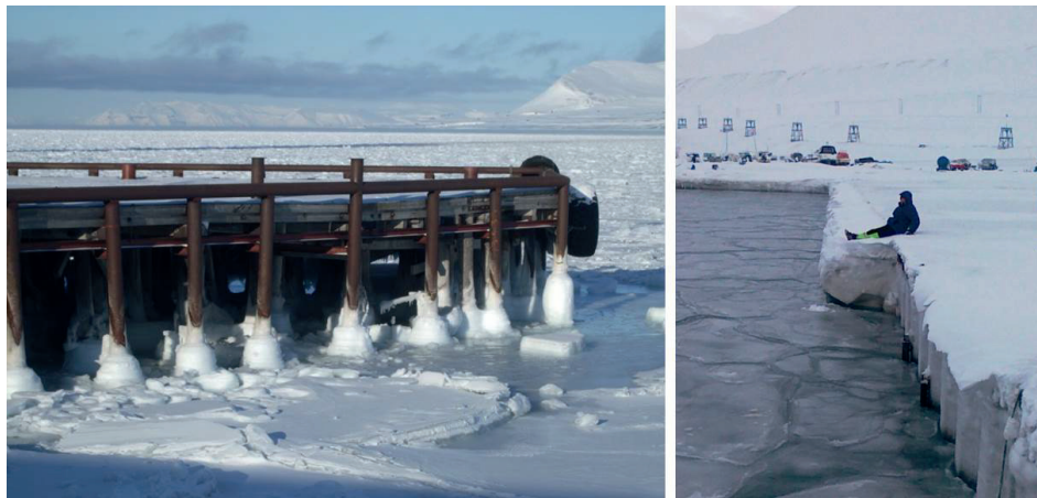
Figure 5.10. Ice accretion on the vertical piles (left) and vertical walls (right).
