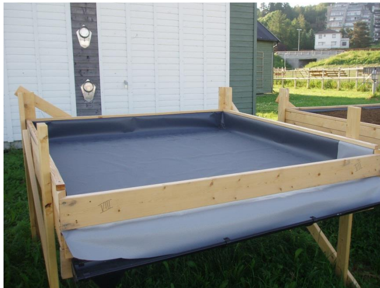
Figure 4. The wooden casket with the protective roof membrane.
