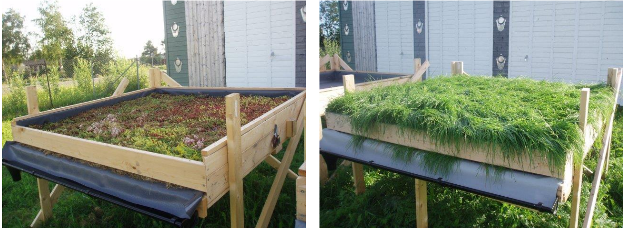
Figure 5. To the left Sedum and to the right Nittledals Roofing Turf® with fully grown grass.
