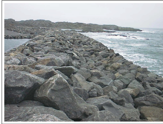
Figure 9.9: The Sirevåg berm breakwater after the storm in January 2002. Source: P. Bruun, 2006
