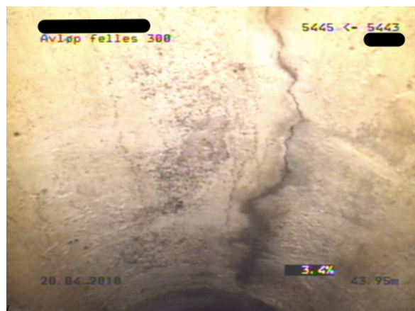
Figure 5.7: 3m longitudinal cracking
