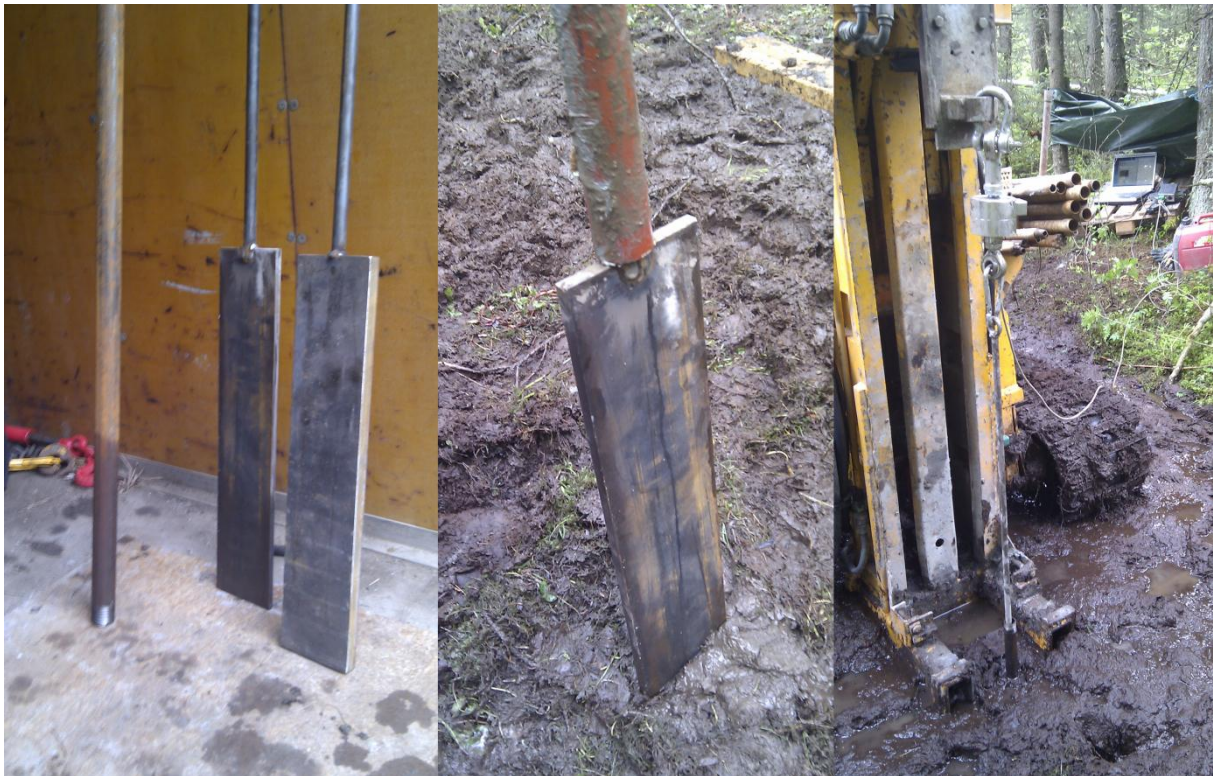
Figure 15 Model test equipment pre-assembled (left hand side), ready for installation (in the middle) and ready for testing (right hand side)
