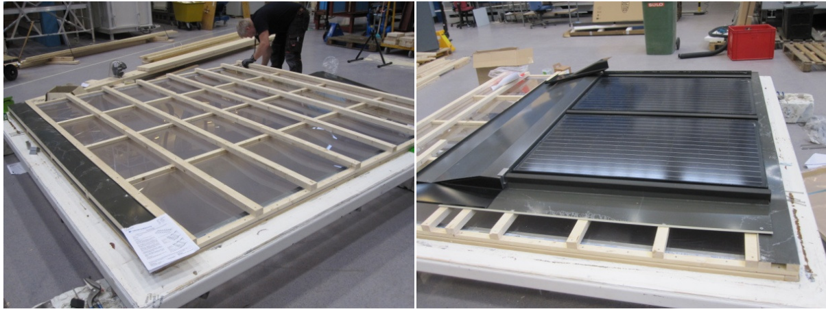
Fig. 2: Roof area with transparent Lexan board wind barrier with double furring strips (left), and the two DuPont Gevity - 165M BIPV modules surrounded by the tailor-made steel fittings from DuPont (right).
