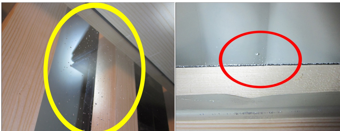
Fig. 8: The droplets of water occurring on the wind barrier, marked with a large yellow ellipse (left), and the water droplets occurring between steel fitting and steel plate roofing, marked with small red ellipse (right).
