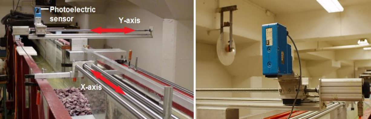
Figure 12-XY profiling system and photoelectric sensor
