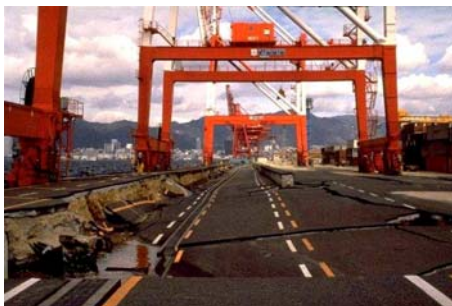
Lateral displacement of a quay wall, Kobe, Japan, 1995
