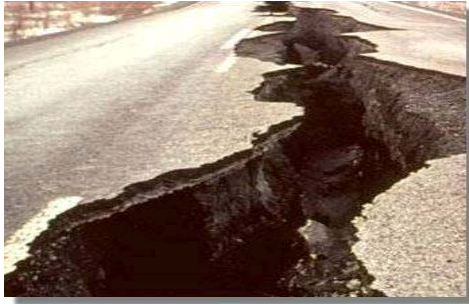
Cracked highway, Alaska, USA, 1964
