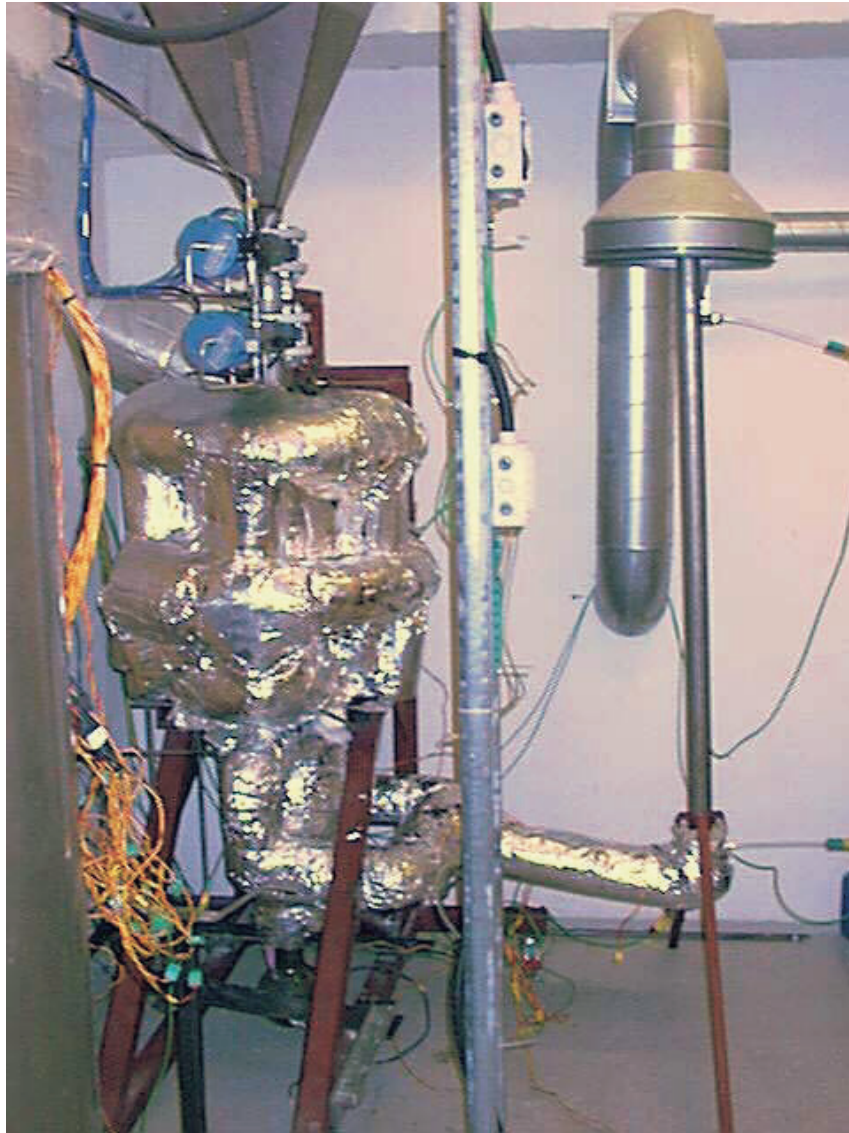
Figure A.5: Stratified downdraft gasifier. Overview
