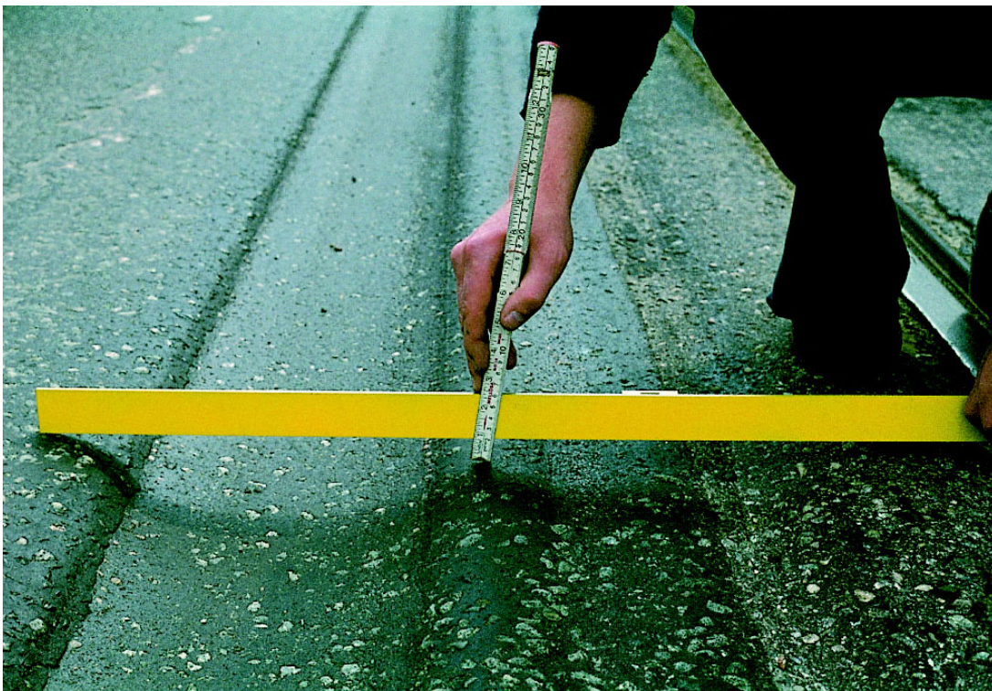
Figure 2.5 Rutting caused mainly by studded tire wear
