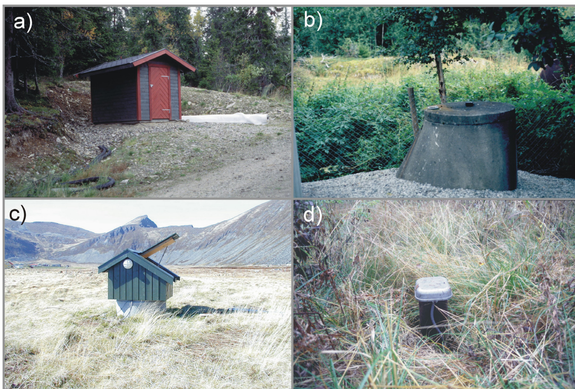
Figure 5.3.2 Examples of wellhead completions. a) Well-house, b) concrete well-protection, c) concrete well-protection with well-cover (small "house") instead of a concrete lid and d) no protection except a proper cap on top of the casing.
