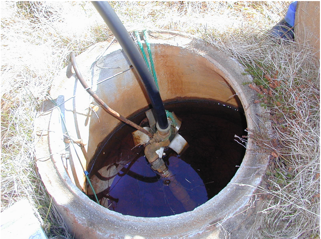
Figure 6.4.2 An example of a well where surface water flows into a leaky concrete wellhead-protection (manhole). In the example the water level periodically exceeds the height of the casing and surface water flows into the well.
