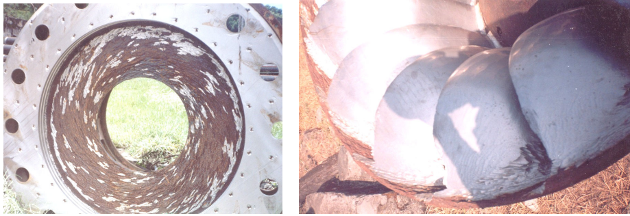
Figure 6.5.2 Photographs of eroded turbine of Sunkoshi hydropower project (left – top cover, right – runner)
