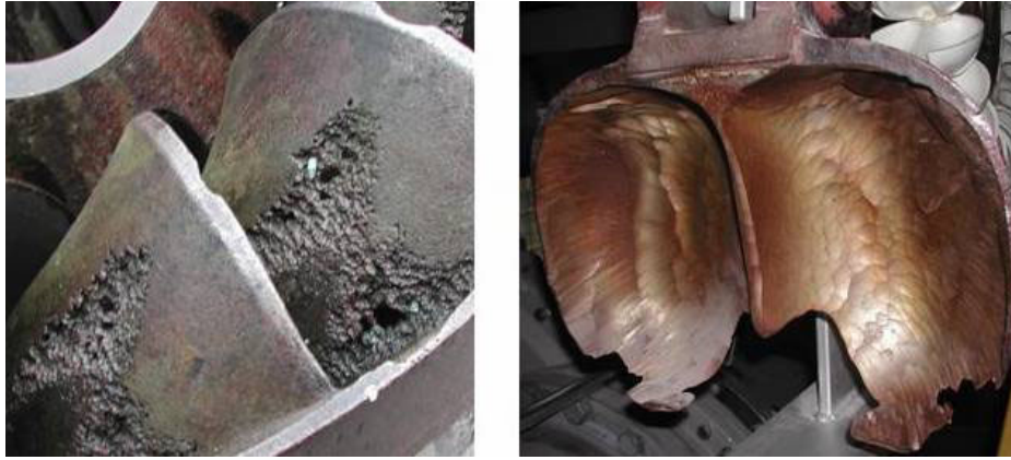
Figure 5.8.1 Pictures of severe cavitation damage in Francis runner (left) and damage of Pelton bucket due to sand erosion (right)
