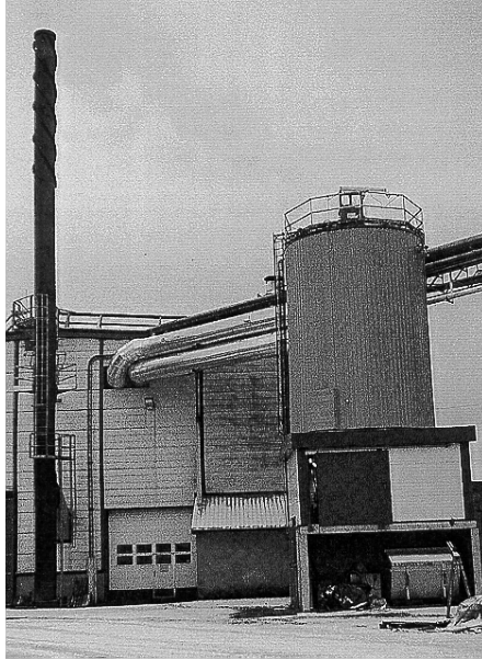
Fig. 9 The commercial scale pilot-plant, capacity of 30,000 m 3 /h. The filter vessel is seen at the right side, with the 5MW boiler house located in the background.
